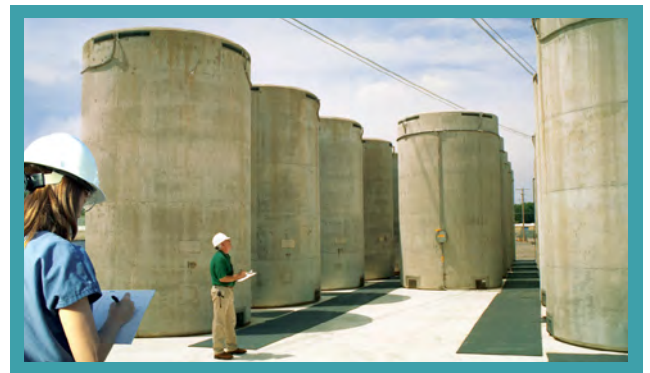
After the cooling period, nuclear energy facilities store used fuel safely on-site in steel and concrete vaults.
